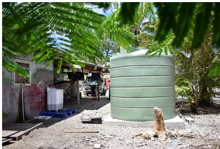
A tank provided by the GCCA+SUPA Project sits on a completed concrete slab at one of the selected households in Nauru
