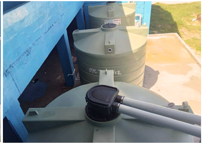
Rainwater harvesting tanks installed at Fetuvalu High School in Funafuti
